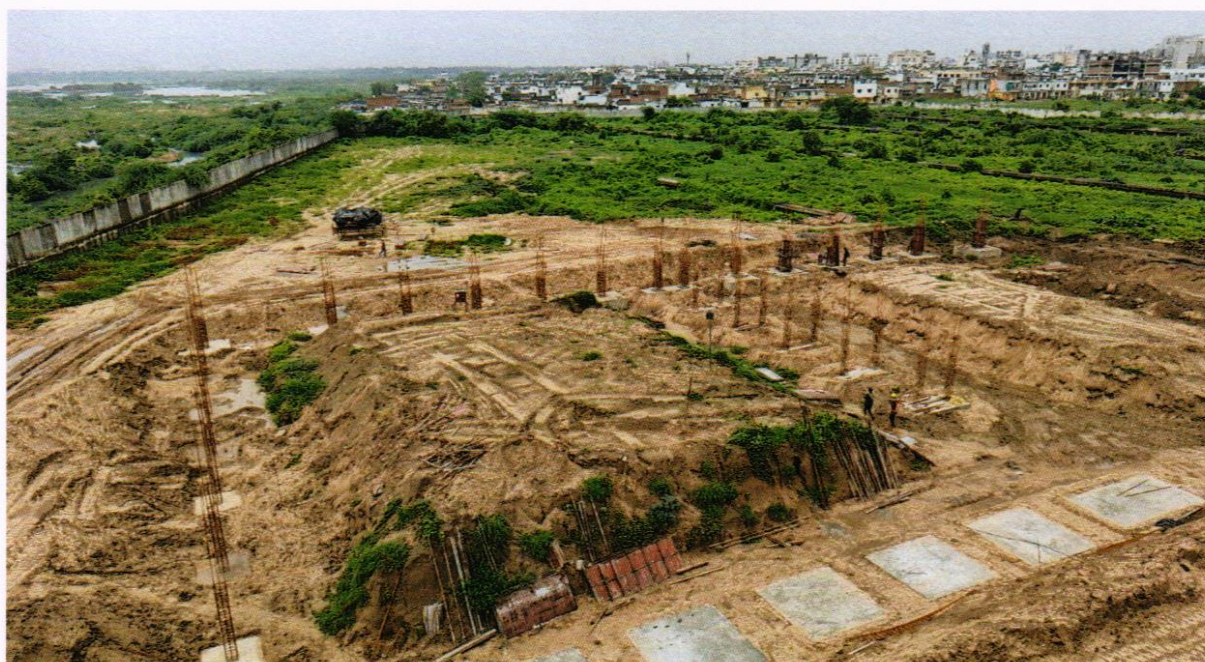
SLUDGE STORAGE PLATFORM
